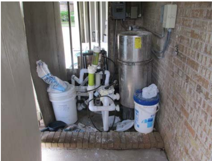
Pool mechanical equipment
