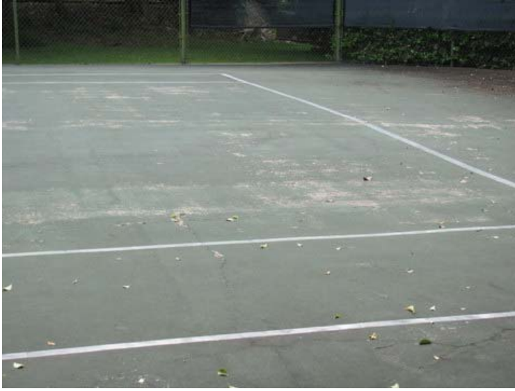
Tennis court surface deterioration
