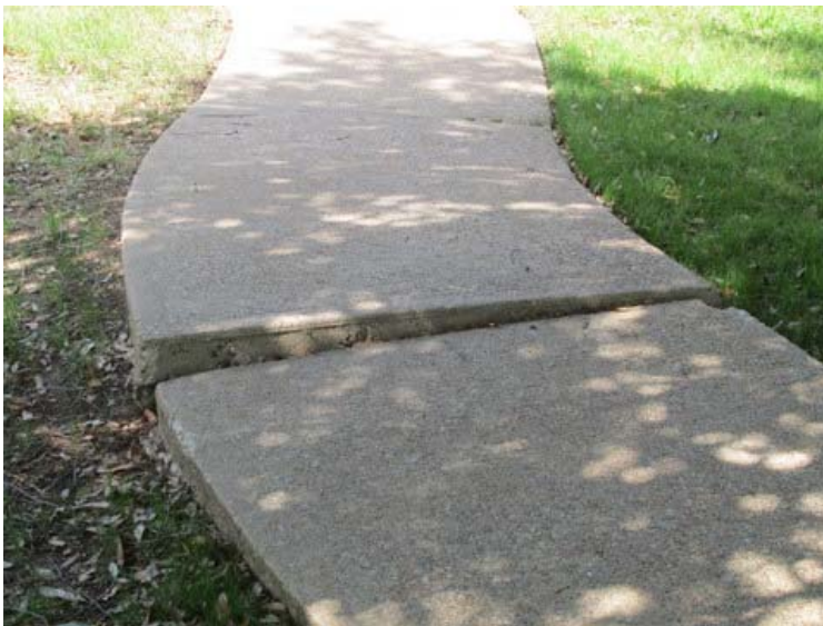
Concrete sidewalk trip hazard
