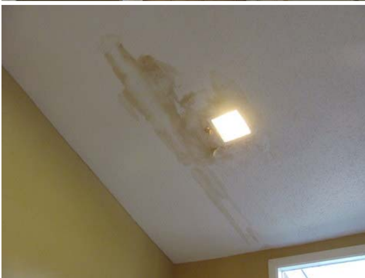
Stain on clubhouse ceiling
