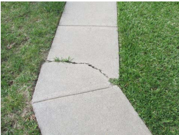
Cracked concrete sidewalk
