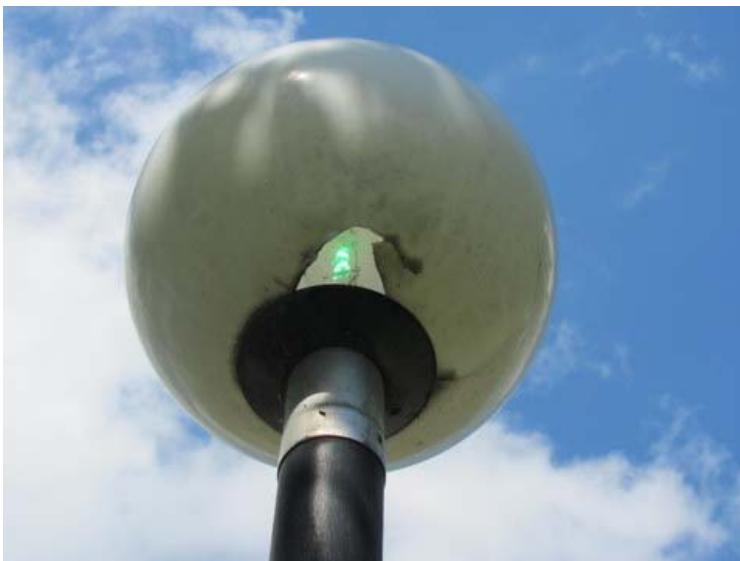
Broken light fixture globe
