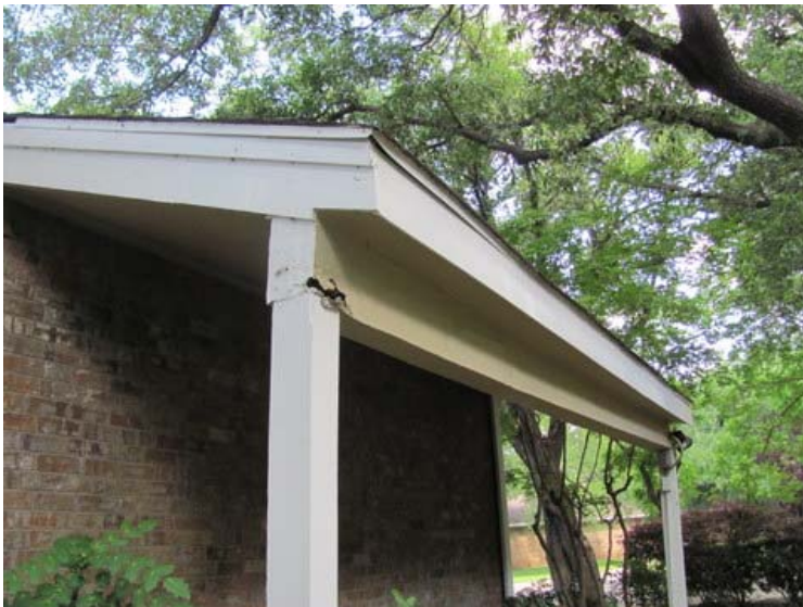
Damage to clubhouse overhang
