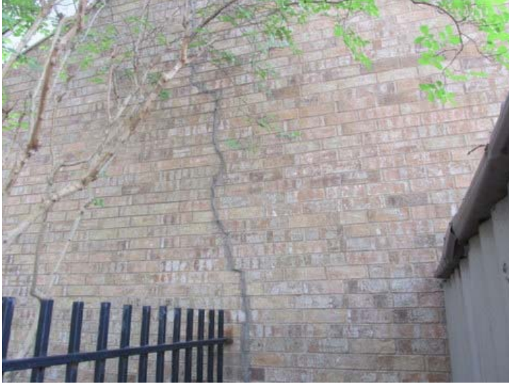
Large crack at clubhouse front wall
