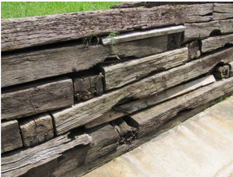
Deterioration at timber retaining wall
