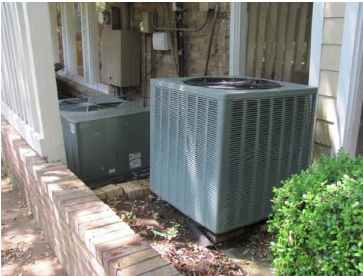
Clubhouse condensing units
