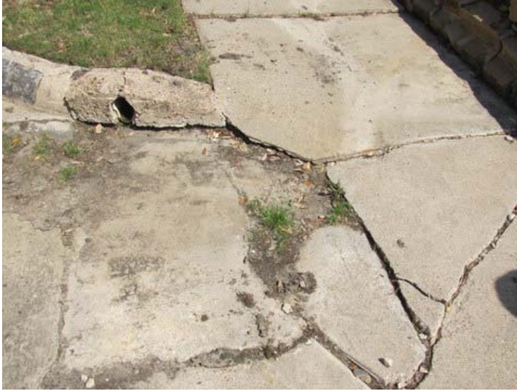
Concrete sidewalk settlement
